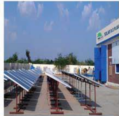
Solar Water Plant
